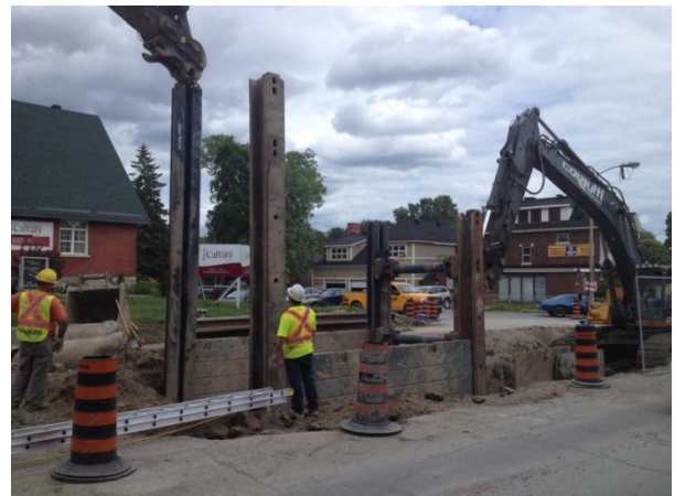
Installation of a trench box to allow work on the 5 m deep storm sewer.
